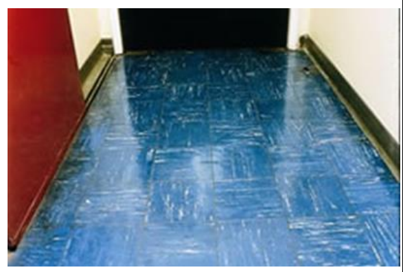
Asbestos containing floor tiles in a corridor
